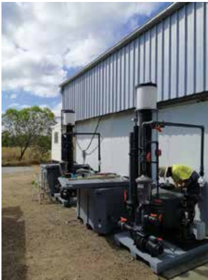
The pumps have been fitted with marine seals that withstand corrosive sea water and filters equipped with marine grade components.
