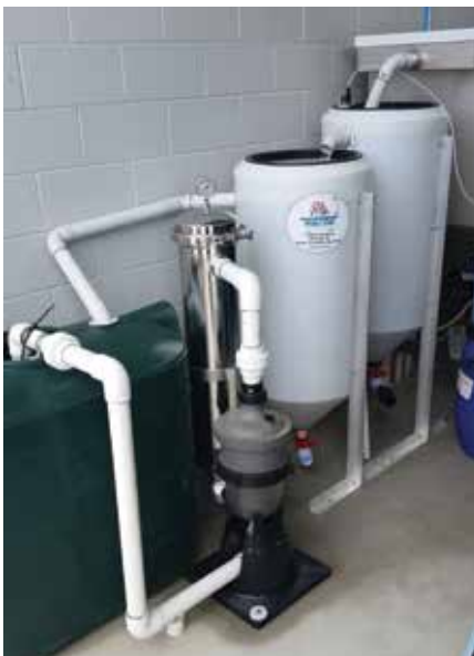
MultiCyclone pre-filters up to 80% of the filter’s incoming dirt load easing the workload of the filter, saving 3,000-litres a week in backwash water.
